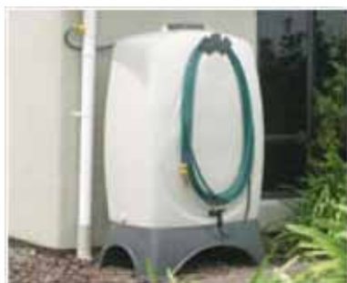
Rain water collection Tank
