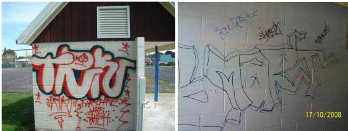
Example of graffiti vandalism – an ongoing problem and cost
