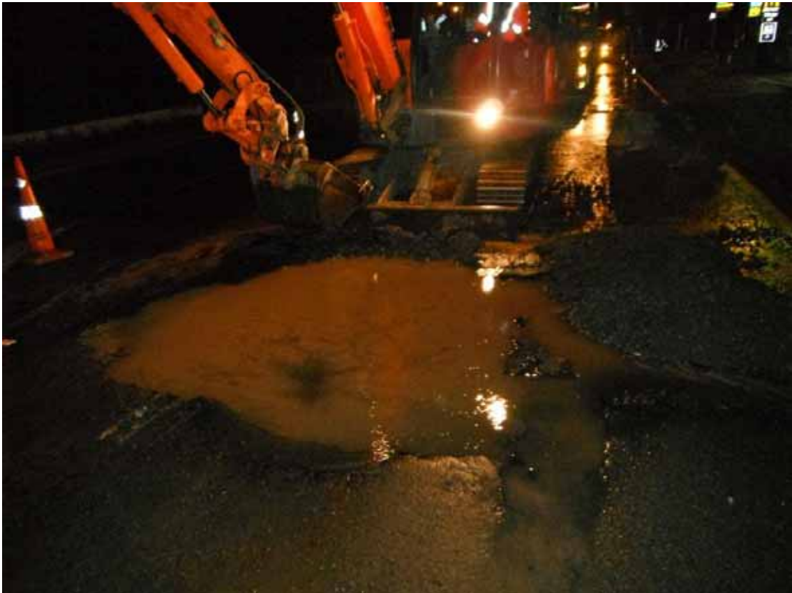
Council contractors at work repairing the water main outside Taumarunui's two 24 hour businesses - McDonalds and the BP on Hakiaha St.
