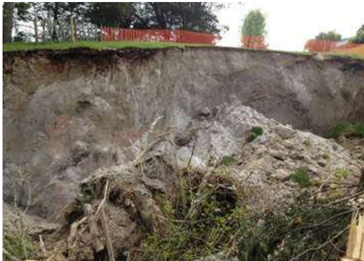
Scour Damage Weston's Water Course
