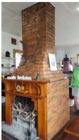
Internal Chimney (1) in shop (Black Chateau Textiles)
