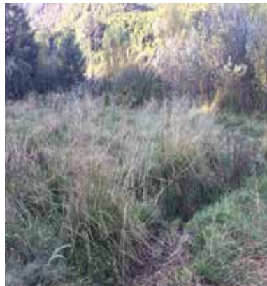
Pipiriki Stormwater – scoured stormwater drain.
