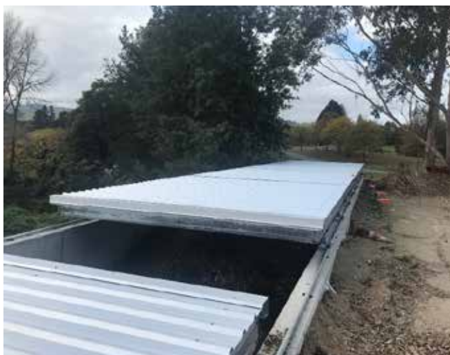
Hot Composting Unit.
