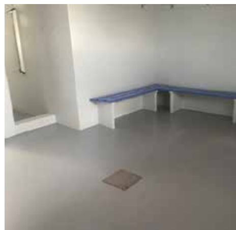
Taumarunui Pool changing room floors.
