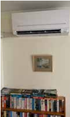
New heatpump at Rochfort Flats, Taumarunui.
