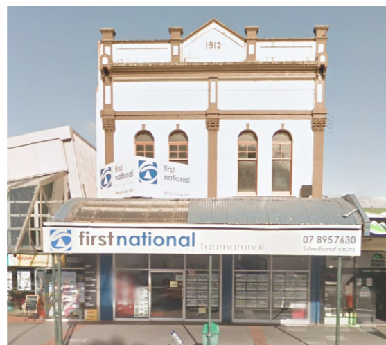
EXAMPLE 2: Strong historical architecture from this 1912 building is being cluttered by signage that hides the architectural features and a verandah's severe pitch which shows too much tin.
