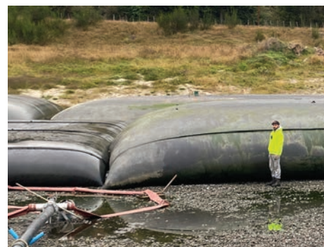
Use of sludge bags has increased performance and capacity of Hikumutu Wastewater Treatment Plant
