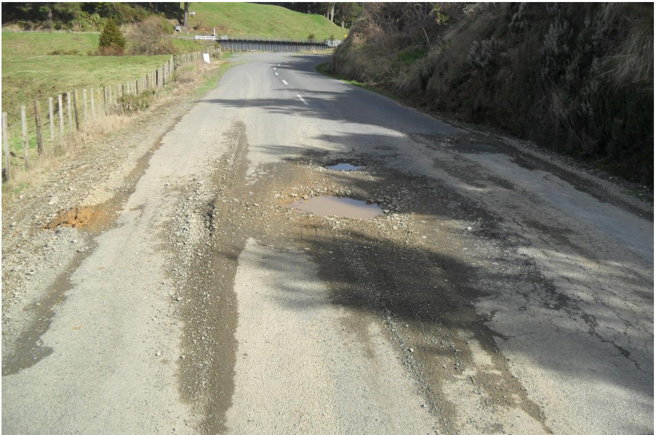
Figure 9 – Sealed Surface Defects on Mangaetuora North Road
