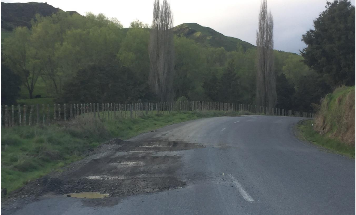
Figure 8 - Sealed Surface Defects on Ongarue Waimiha and Poro O Tarao Roads
