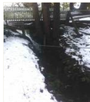
Choke in Miro Street watercourse - tributary in Ohakune
