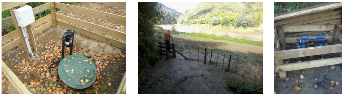
New WWPS (left), irrigation field (middle), control valves for the distribution through the irrigation field (right)
