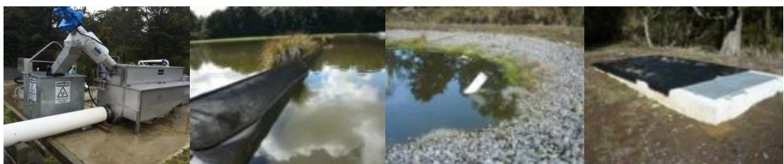
Grit & solids removal (left), Stop log wall between primary and secondary oxidation lagoons (2 nd from left), Tertiary stone media lagoon (3 rd from left), UV Disinfection chamber (right)
