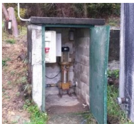
Sunshine Road Booster WPS, Taumarunui (for future dosing if required)
