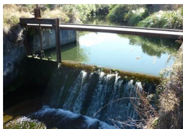
Ohakune Raw Water Intake
