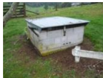
Te Peka Booster WPS, Taumarunui
