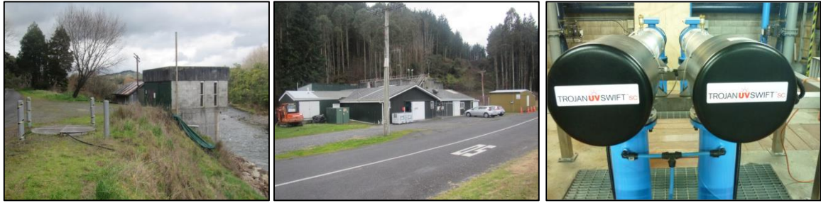
Water intake (left), Taumarunui WTP (middle), UV disinfection units (right)
