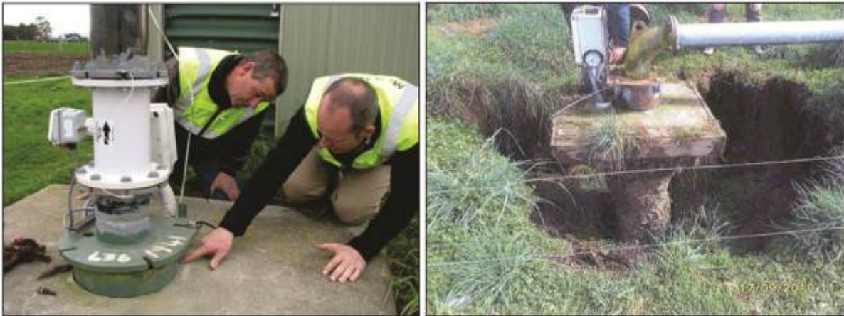
Figure 3.13: Examples of damage to wells caused by the M_w 7.1 earthquake. Some well heads rose out of the ground, while others were affected by settling/subsidence around the annulus (photos supplied by H. Rutter, Aqualinc, via Zemansky et al. , 2012).
